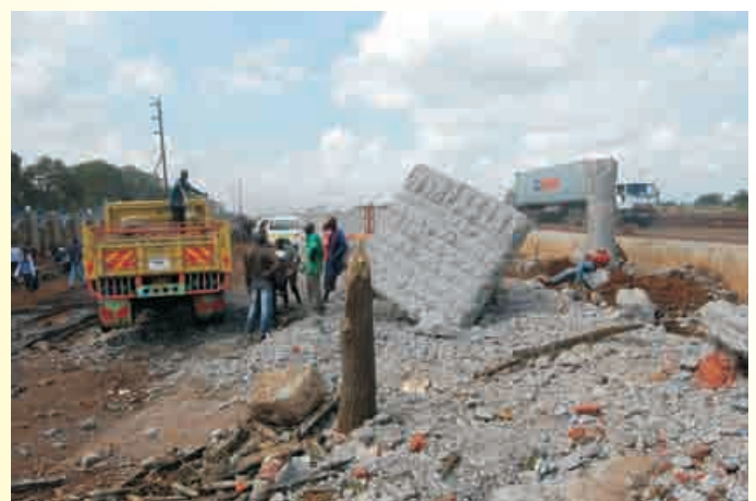
Workers bring down the 'KU Bridge' on Thika Road as part of the ongoing construction of the superhighway.
